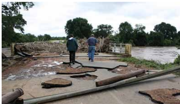
Damage to the Nwanedzi Bridge after flooding.
