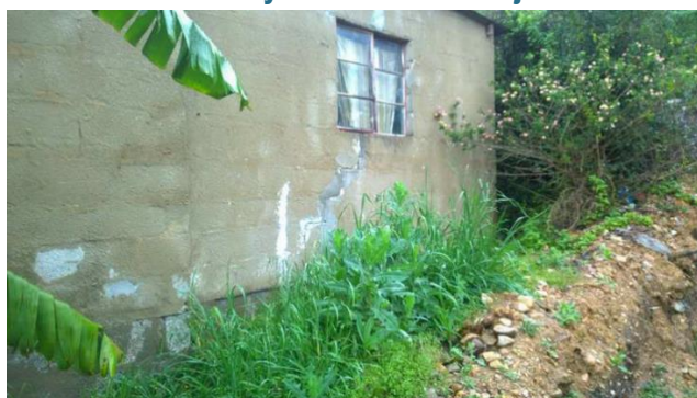
Figure 2: Damages caused by mudslides caused by poor floods in Wittedrift
